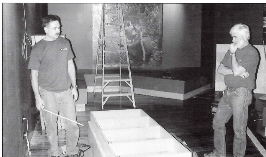
Construction in progress as the new gallery space is prepared for "Uncovering the Enemy" exhibit.
